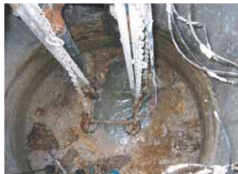
Before: pump station has a rancid grease cap
